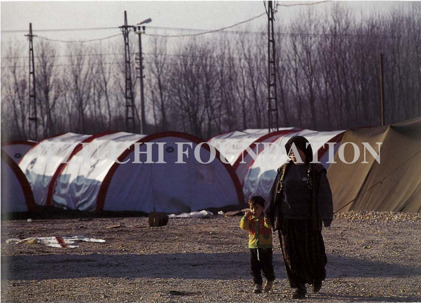
Through severe weather and more earthquakes, two hundred large insulated tents were completed after two months of continuous work, just before the end of Ramadan, the Islamic month of fasting.
